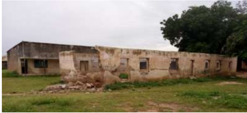
Plate 1: Dilapidated Classrooms in Ganye Town, Ganye LGA.
